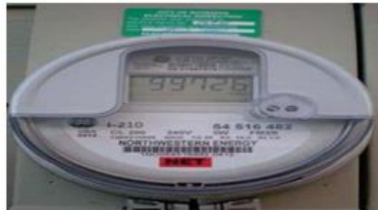
Fig 7.6 Smart Meter appliance
